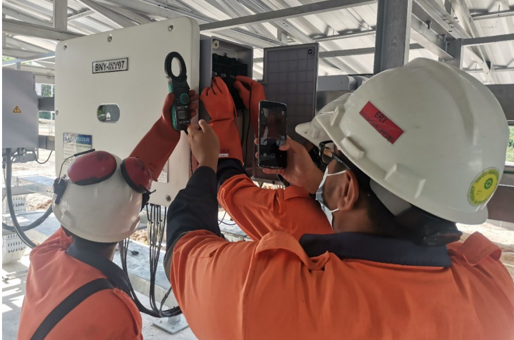
Ground Shot of Solar Hybrid Power Plant for self-consumption at an Indonesian mining site
